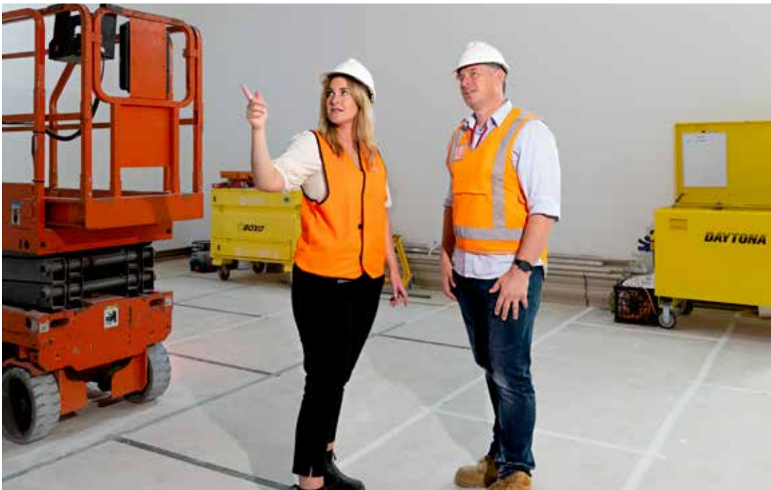
Project Manager Kacie O'Sullivan and Site Manager Peter O'Connor inspecting the LED project at the National Gallery
