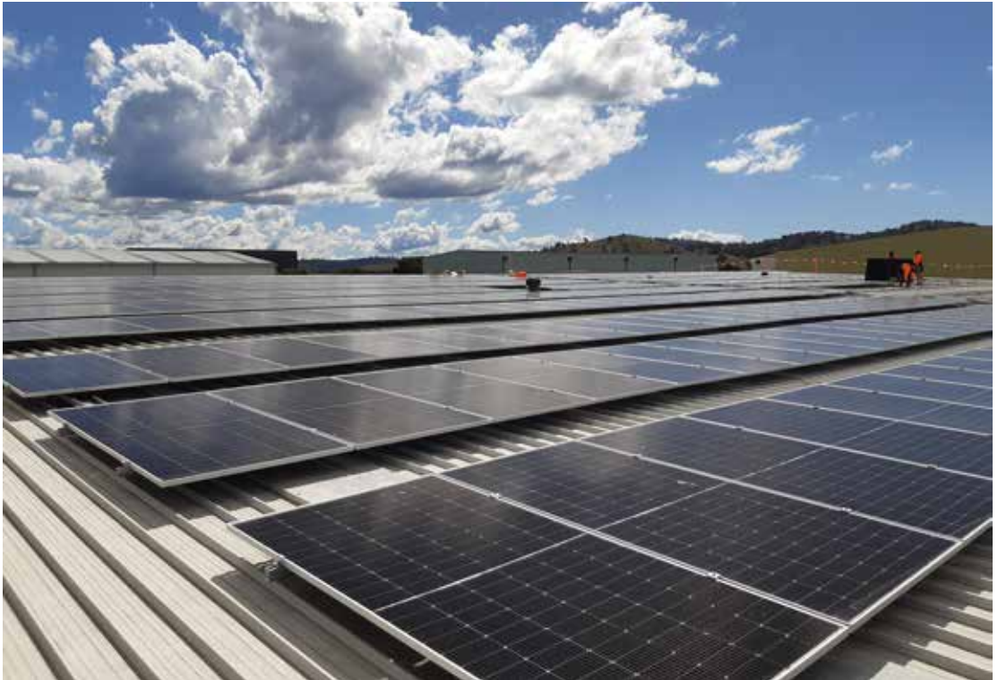
The Solar Project: solar panels at the National Gallery's offsite storage facility
